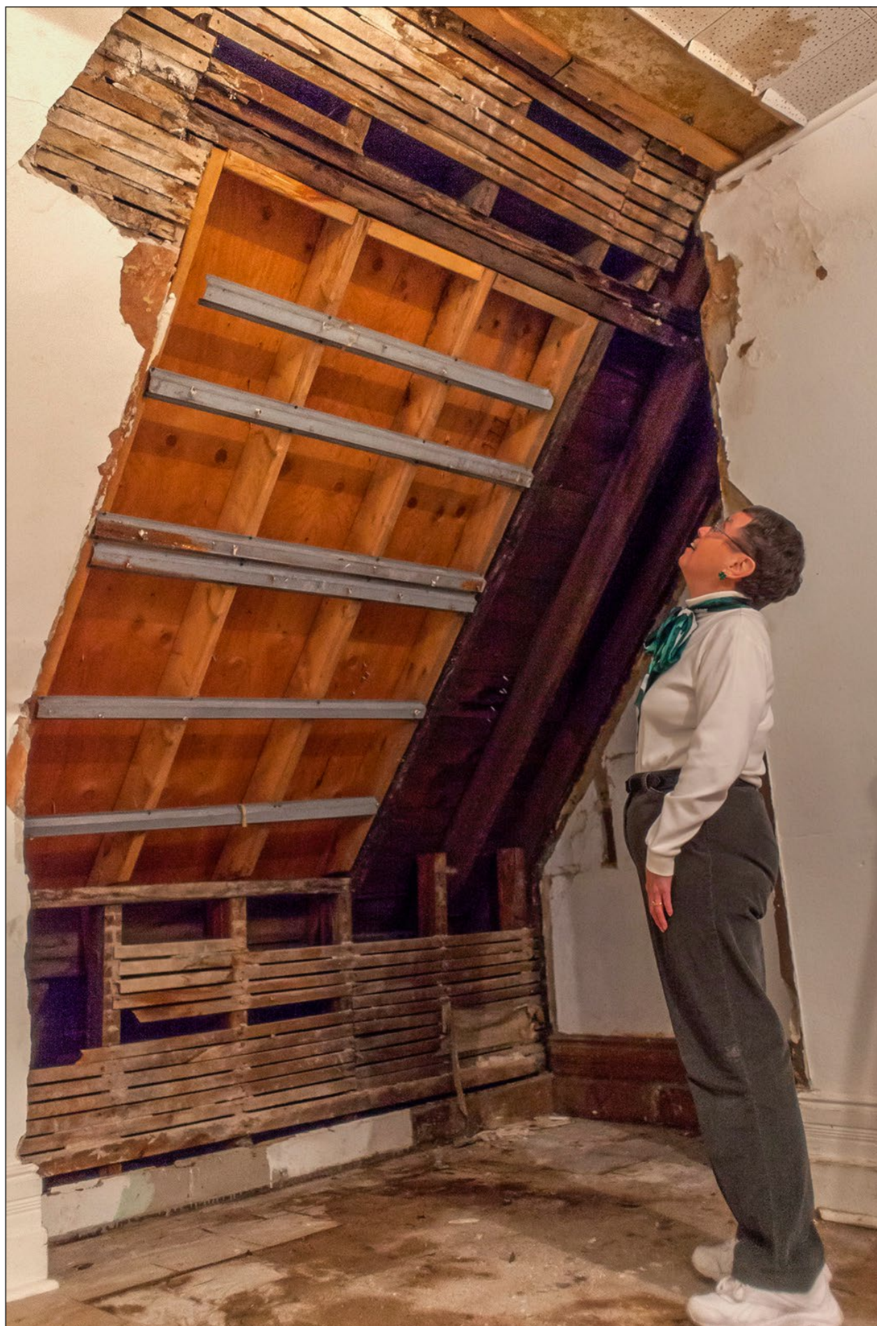
Judy Ducommun, member of the finance and maintenance committee for St. Andrew's Presbyterian Church, looks over the damage after freezing rain and a thaw caused water damage to the wall and roof of the church storage room.
