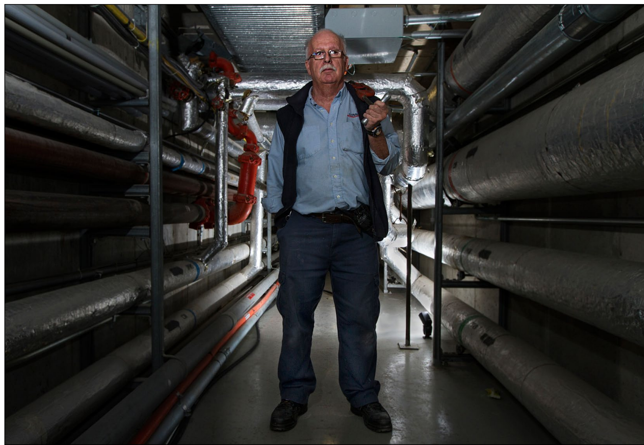
Stephen Glover has been a plumber since 1974, and is currently a commercial plumber at Loyalist College. March 11 marks the fifth annual World Plumbing Day, a day of awareness for the public to better understand what these tradesmen do for their community.
